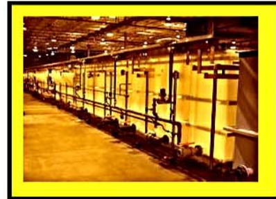
TANKS IN SERVICE
