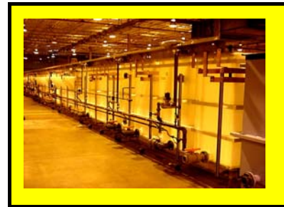
TANKS IN SERVICE
