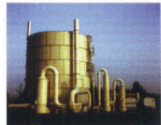
H2S/AMMONIA ODOR CONTROL SCRUBBERS
