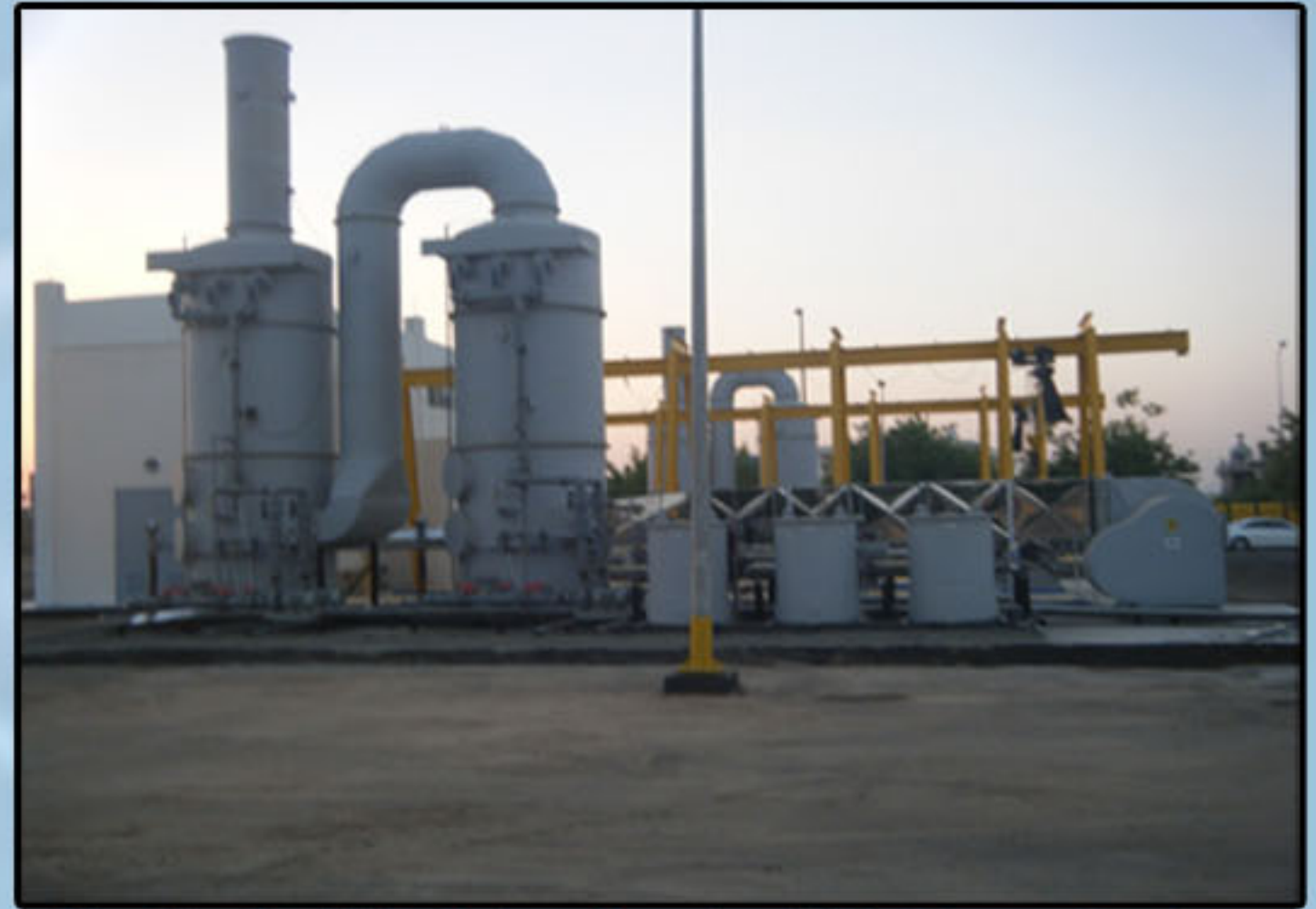
Vertical - H 2 S Odor Control (2) Stage System
